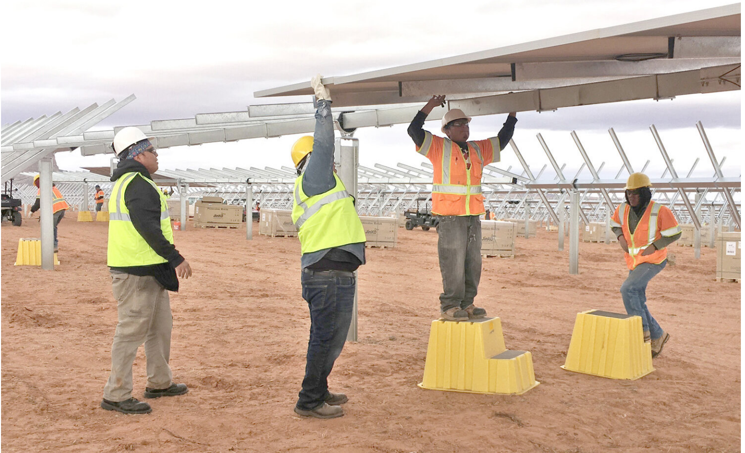
A Navajo Tribal Utility Authority crew installs solar panels (Courtesy: Navajo Tribal Utility Authority)
